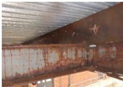
Evaluation of corroded structural steel framing elements
